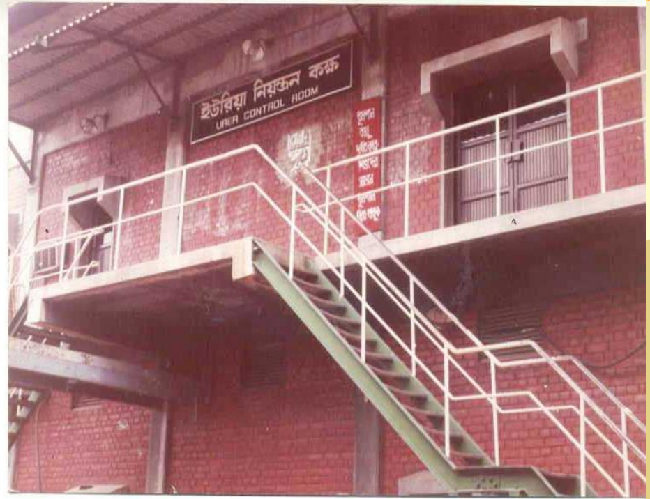
Control room was 21 m away from the stripper, was on the second floor and with single exit stair
